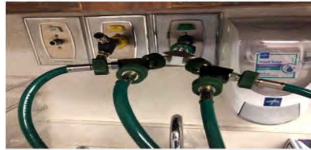
Figure 1A: One wall oxygen outlet being split into four pipeline supplies through the use of three Y-piece splitters.
